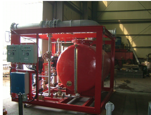
Foam Pump Skid
