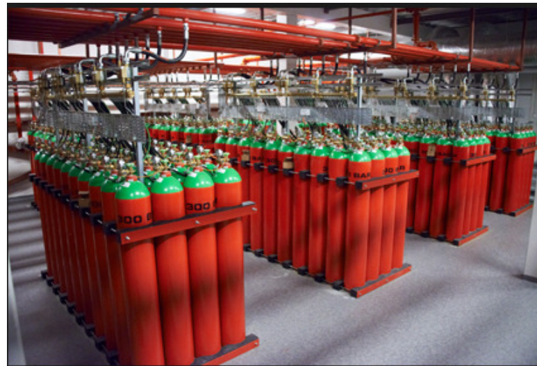
Inergen Skid (300bar)
