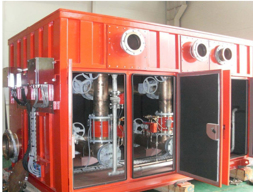
Deluge Valve Skid
