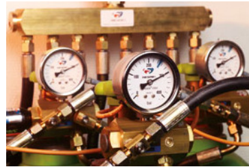
Pressure Gauge and Manifold
